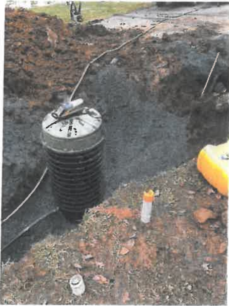
Typical grinder pump installation
