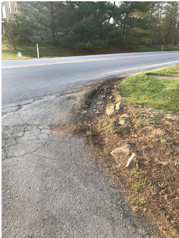
PICTURE #2 - Shows pavement distress, no shoulders, tight radii and vehicular off-tracking.
