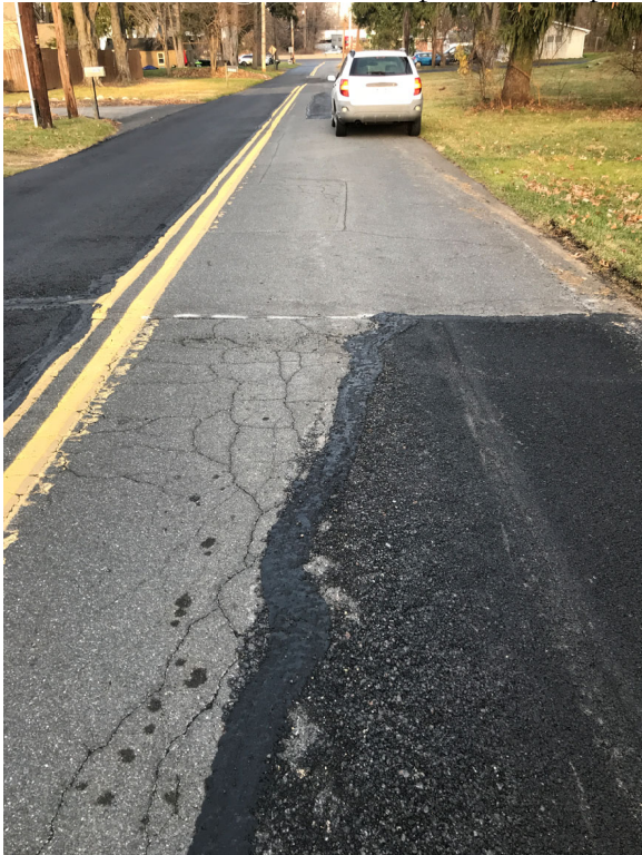
PICTURE #4 - Shows pavement distress, no shoulders and pavement repair.
