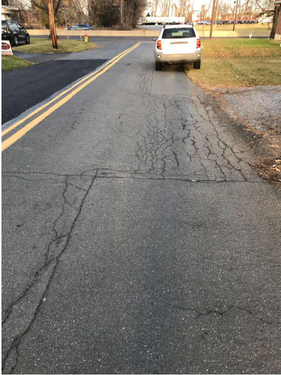
PICTURE #3 - Shows pavement distress, no shoulders and pavement repair.
