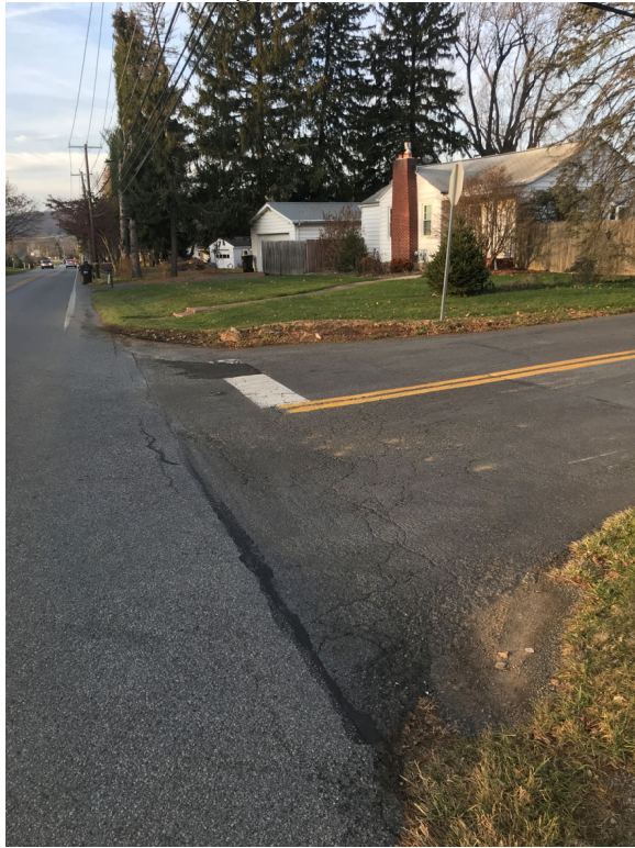
PICTURE #1 - Shows pavement distress, no shoulders, tight radii and vehicular off-tracking.
